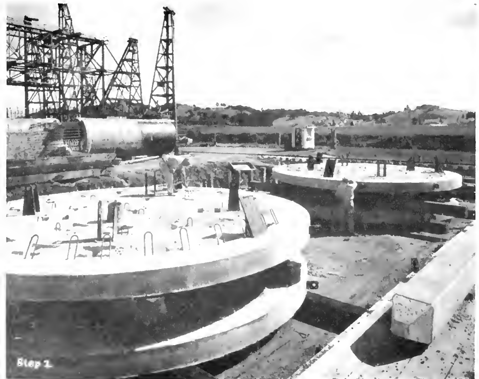
STEP 2—Precast base grid for Pier 54 in place on barge for transportation to bridge location
